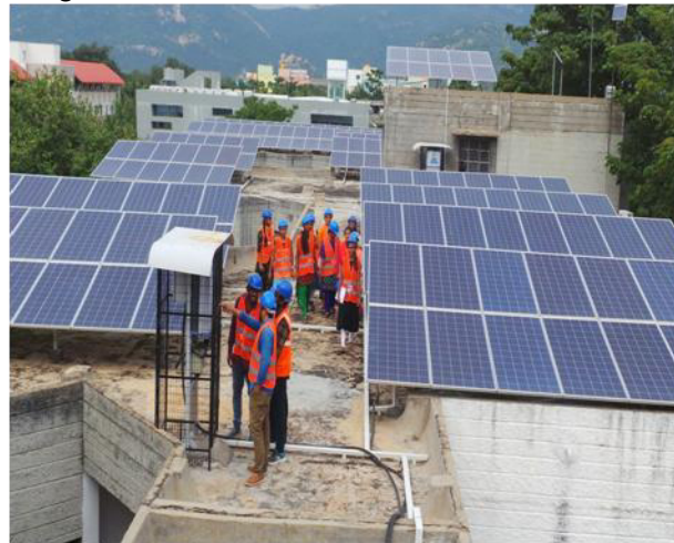
Roof top Solar PV System (500kW)
