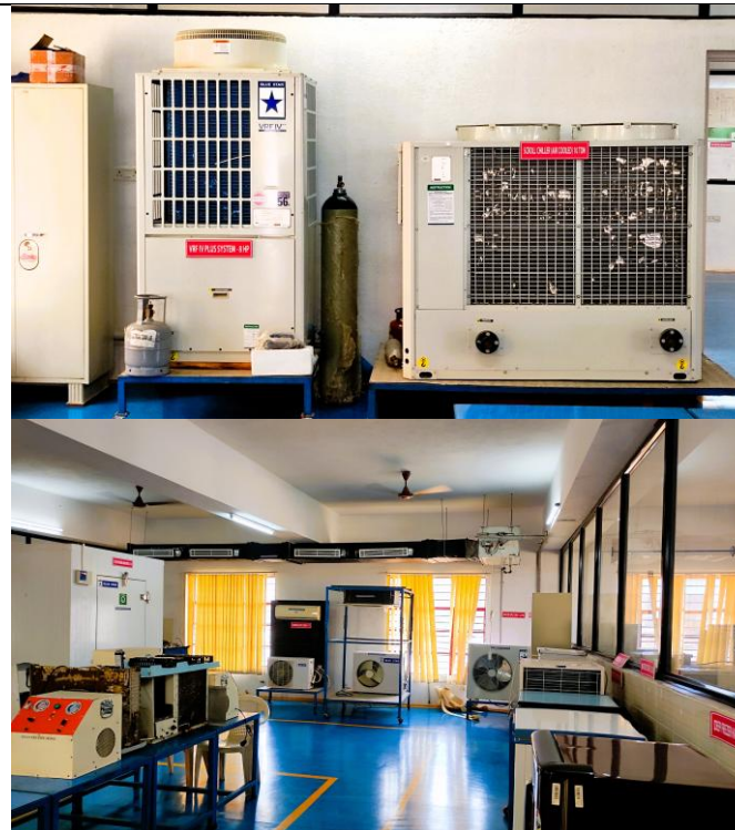
HVAC Setup Room No. 4A
